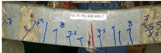
(a) Flexure failure
