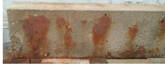
(b) Vertical cracks
