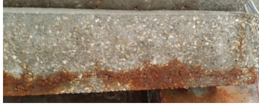
Fig. 4: (a) horizontal cracks
