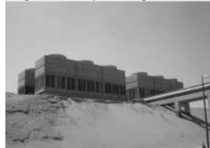
Fig. 15. Cooling towers at AUC's central utility plant.[36]
